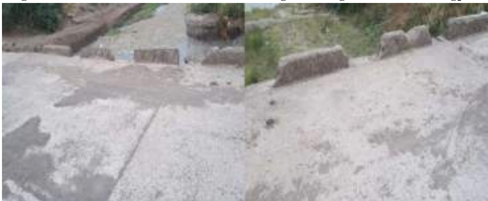
Figure 6: Damage Wheel Guard and Reflectors
